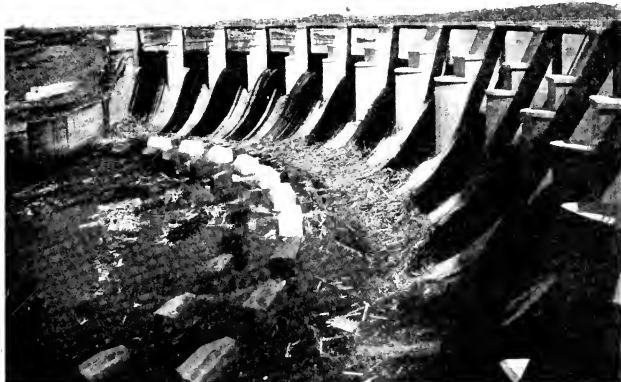
FIG. 4. GATUN SPILLWAY DAM. BAFFLE PIERS IN FOREGROUND. ENTRANCE TO MACHINERY TUNNEL IN DISTANCE.
